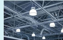
Efficient lighting system
