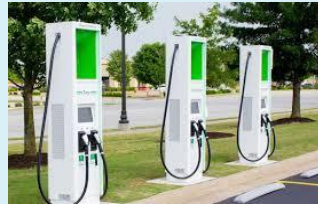
Parking lot with fast EV chargers
