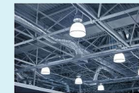
Efficient lighting system
