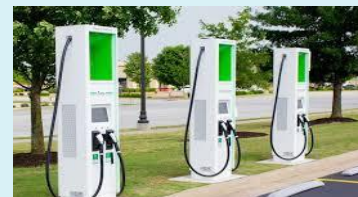
Parking lot with fast EV chargers
